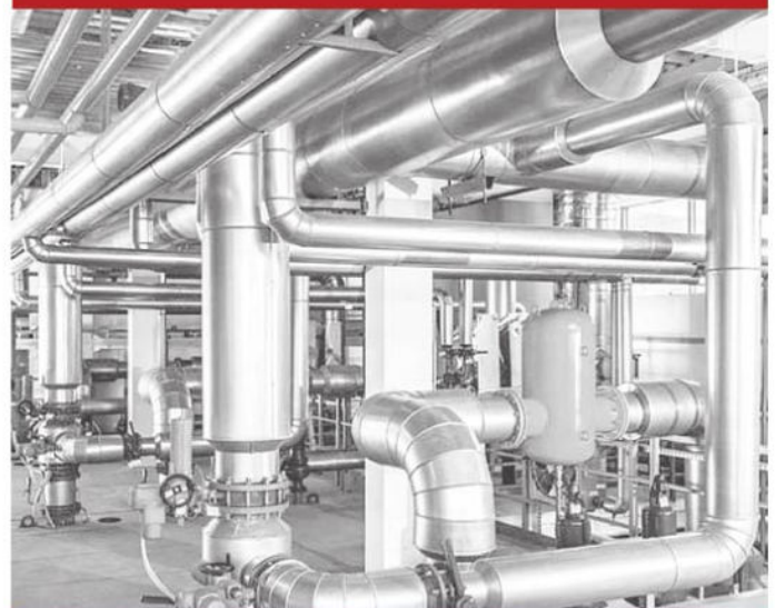
PROCESS UTILITY SYSTEM
